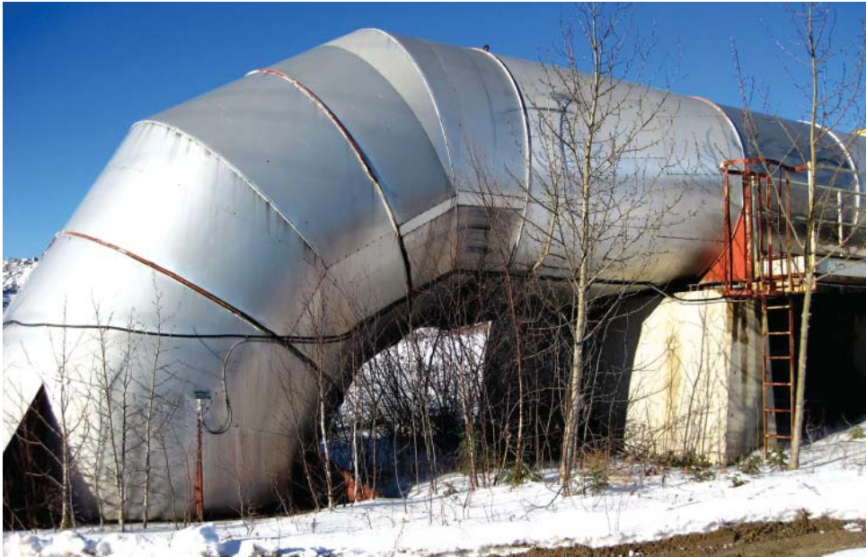
Stantec conducts a detailed engineering study on the ventilation waste heat recovery system of a large, remote, underground mine. The study leads to an upgrade project that paid for itself within a year. (Photo: Stantec)
