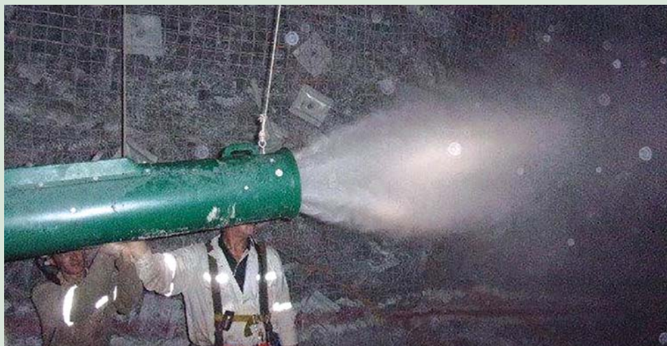
Water in the hole! The MOUSETRAP Atomizer, which is blast instigated and has a timed shutoff, broadcasts a cloud of atomized water that binds to microscopic dust particles that then rain down, cleaning the air and area. (Photo: Terramin)
