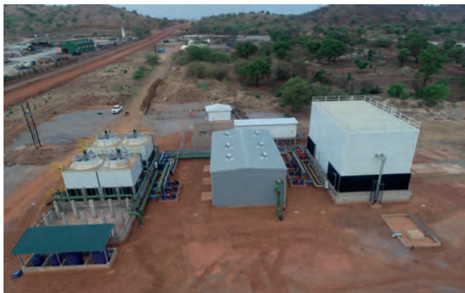
Howden recently delivered the first phase of a 8 MW surface bulk air cooling plant for Roxgold's Yaramoko gold mine in Burkina Faso
