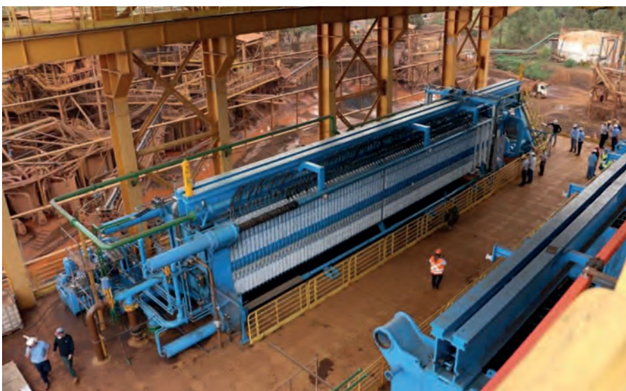
ANDRITZ overhead filter presses A4 F 2500 with a future-proof control and automation system for tailings treatment (© IMAGINE IMAGENS INCRÍVEIS)
